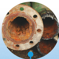
Clogged rusted pipe
